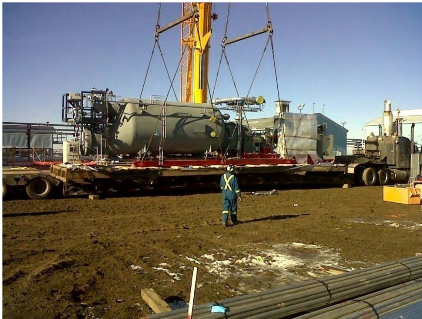
ORC Skid Lift
